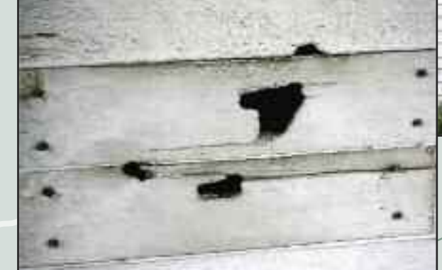
The Cannon Ball House in Blountville still shows shell damage to the exterior claphoard in the rear of the house.
